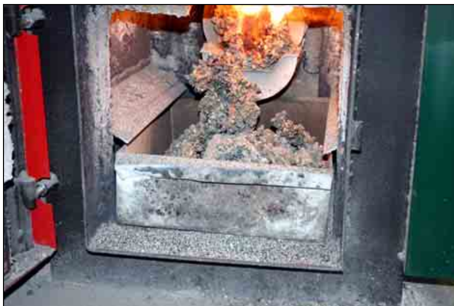
Changing quality of bio-pellets and improper kettle for its combustion can cause unpleasant effects. On the picture - Ash clinkering in the area of the burner and cinder pocket.
